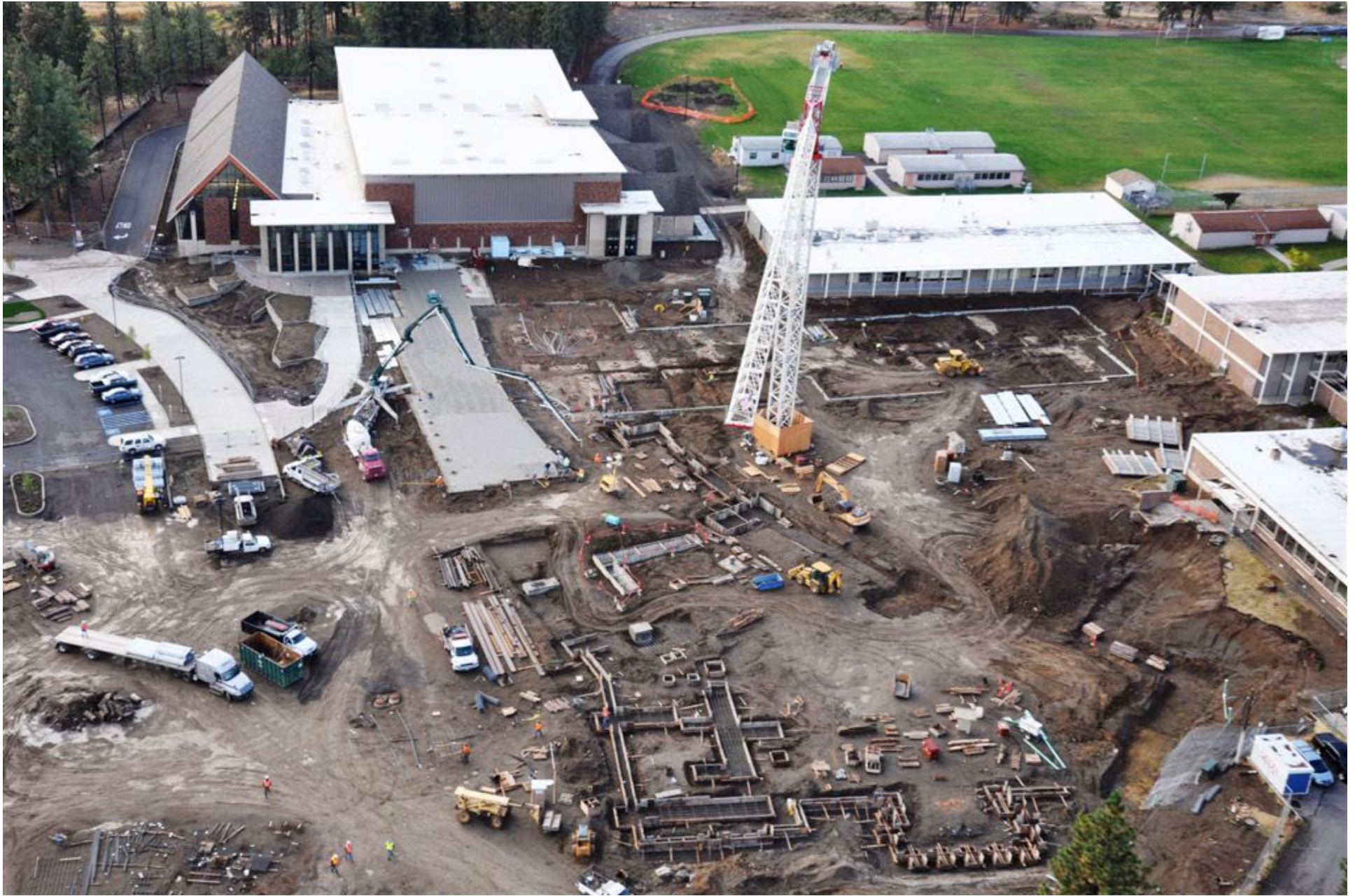
Construction moves along on the Ferris High School modernization project. Watch the progress on the Ferris webcam.
